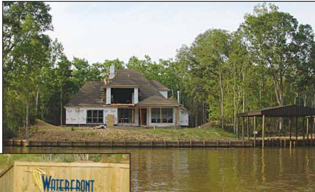
Total privacy awaits new residents of a home under construction in the exclusive WaterFront Sanctuary development in Maurepas.
